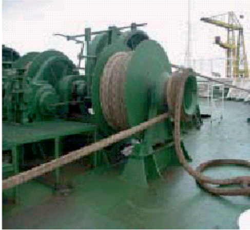
Figure no. 8: Mooring line on the tensioning part of the winch drum
